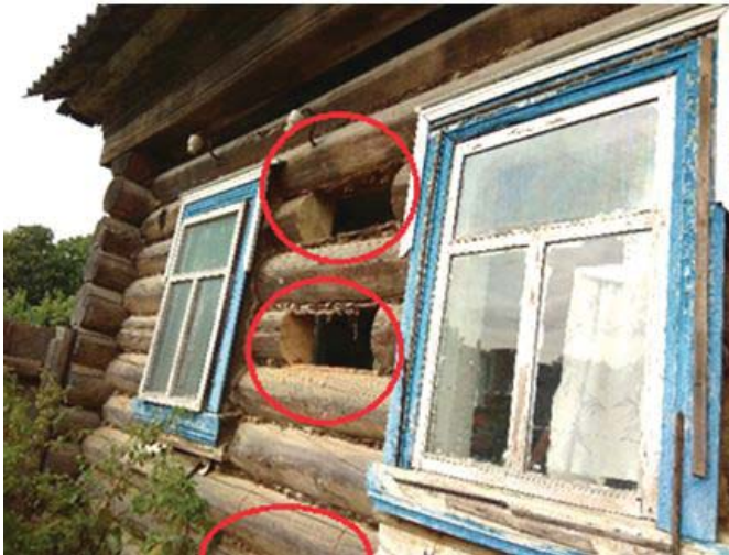
Figure 6: The south side of the house (red ovals mark the places for selecting shock bolt-fragments for test samples)
